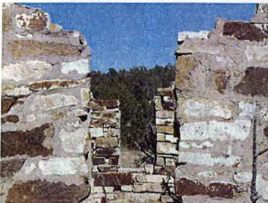
5LA.11809 the exterior of this dwelling has been repointed with concrete but the original adobe mortar is still visible on the interior
