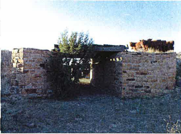
5LA.11788. Bridge located on the original route of the Trinidad Highway (now Highway 106)
