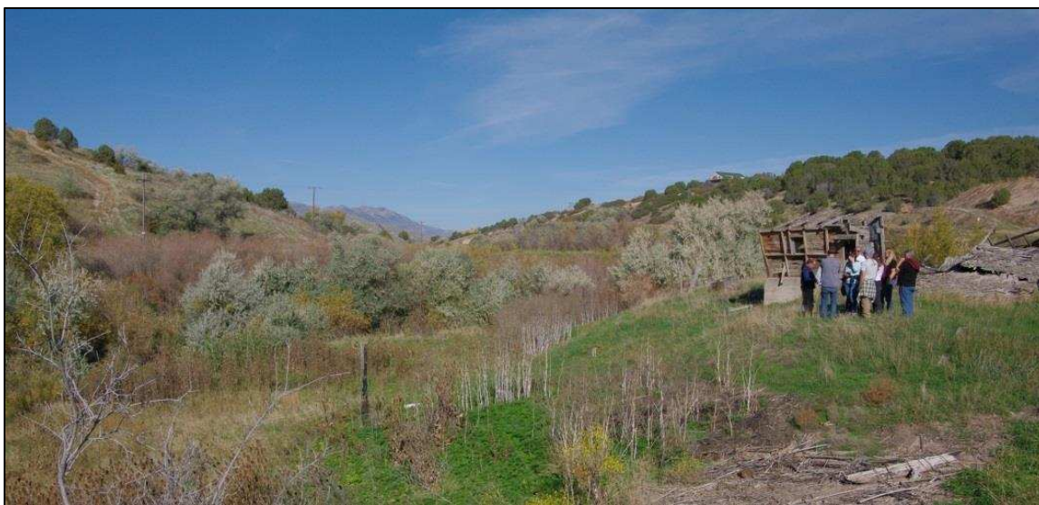
Figure 4.15: Contemporary earthen aqueduct that conveys the West Cache Canal across Battle Creek. A small culvert in the base allows the creek remnant to trickle downstream. The original aqueduct was built between 1898-1904, then blew out in the flood of 1911. It was rebuilt after that. These construction episodes probably directly impacted the Shoshone village remnants.
