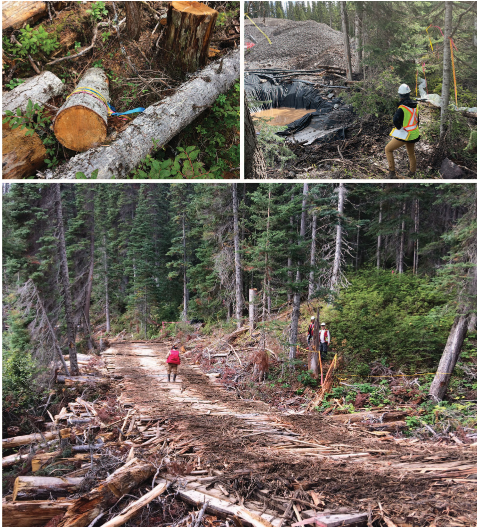
FIGURE 5 Culturally modified trees with blaze scars felled by construction crews. Consultant archaeologist observes destruction of Kweese War Trail (flagged on right) beside Coastal GasLink road construction in 2022. Pipeline road built over sections of the Kweese War Trail in 2020; note aurhots Ridsdale and Spice (right) on small segment that survived the construction but will ultimately be obscured from brushing. (Photograph by Chelsey Geralda Armstrong) [This figure appears in color in the online issue]
