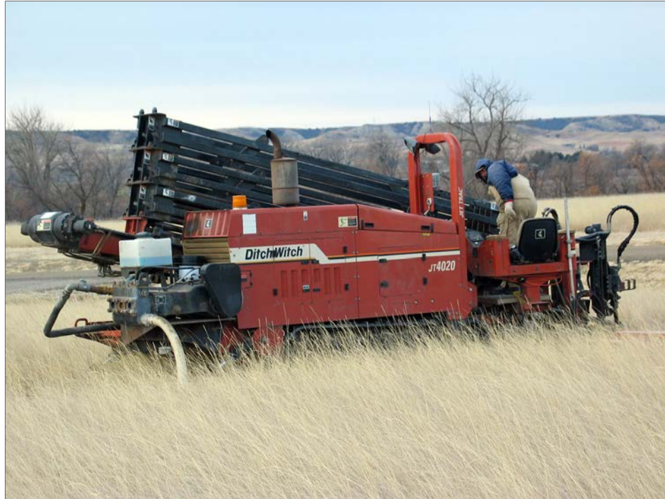
a) view of Ditch Witch JT 4020 all terrain directional drilling rig (view to the southwest)
