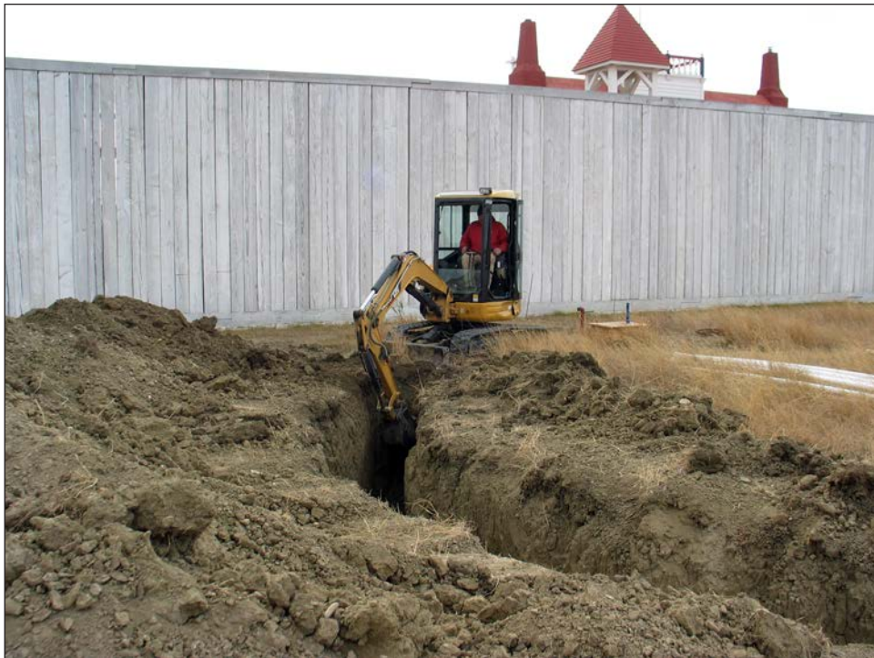
Figure 32. Excavation of the trench for bypass of the 500 gallon fire suppression storage tank (view to the southwest).
