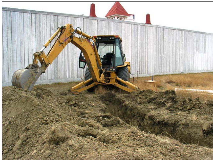
Figure 28. Caterpillar 420D backhoe loader in operation along outside of North Palisade Wall (view to southwest).
