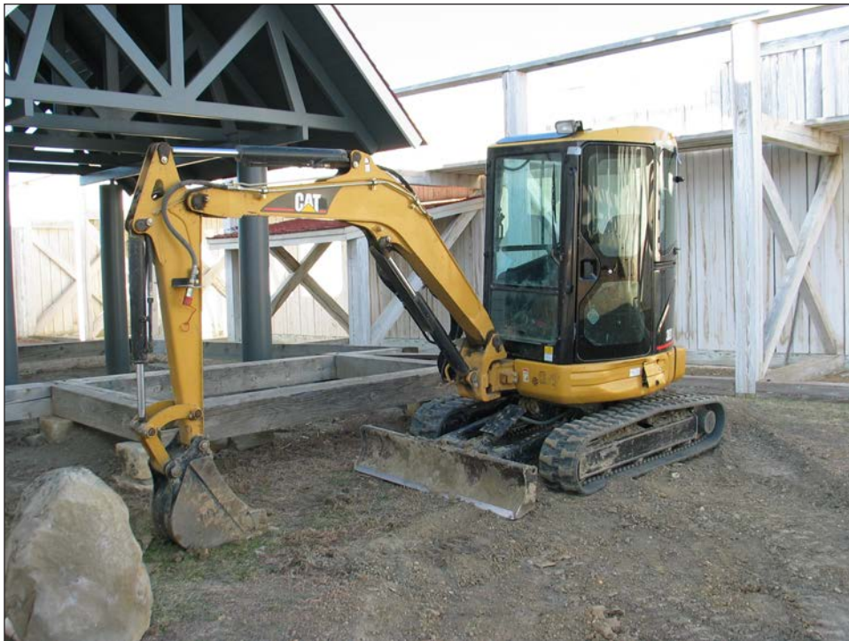
Figure 29. Caterpillar 303 CR mini hydraulic excavator in operation next to the east side of the kitchen (view to the southeast).
