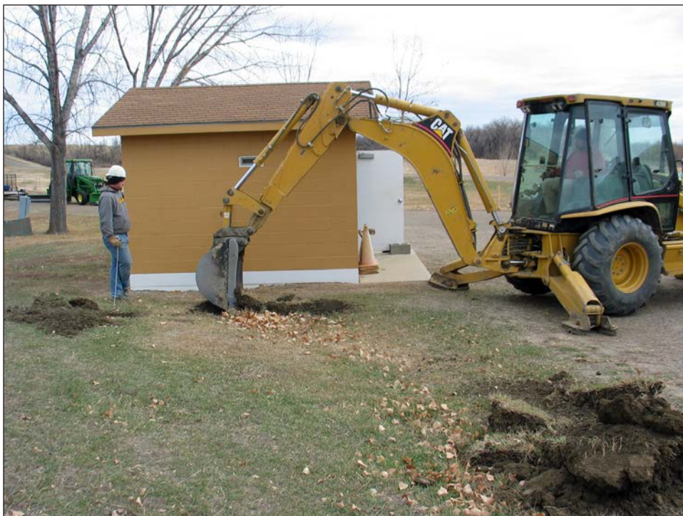
Figure 35. Excavation of trench next to west side of well house at Site 32WI996 (view to the east).
