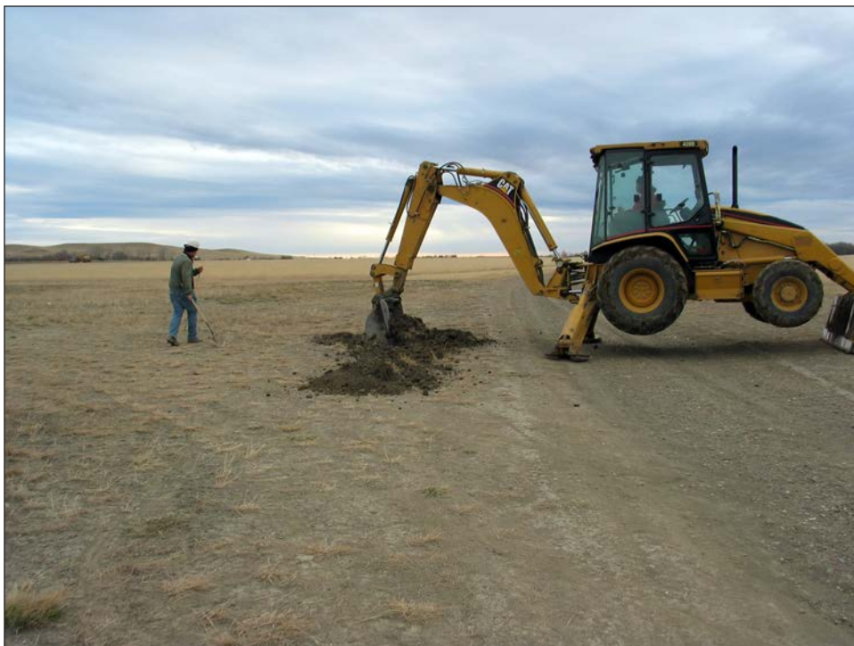
Figure 38. Excavation of existing waterline trench in Grid Area 2 next to park service road (view to the east).
