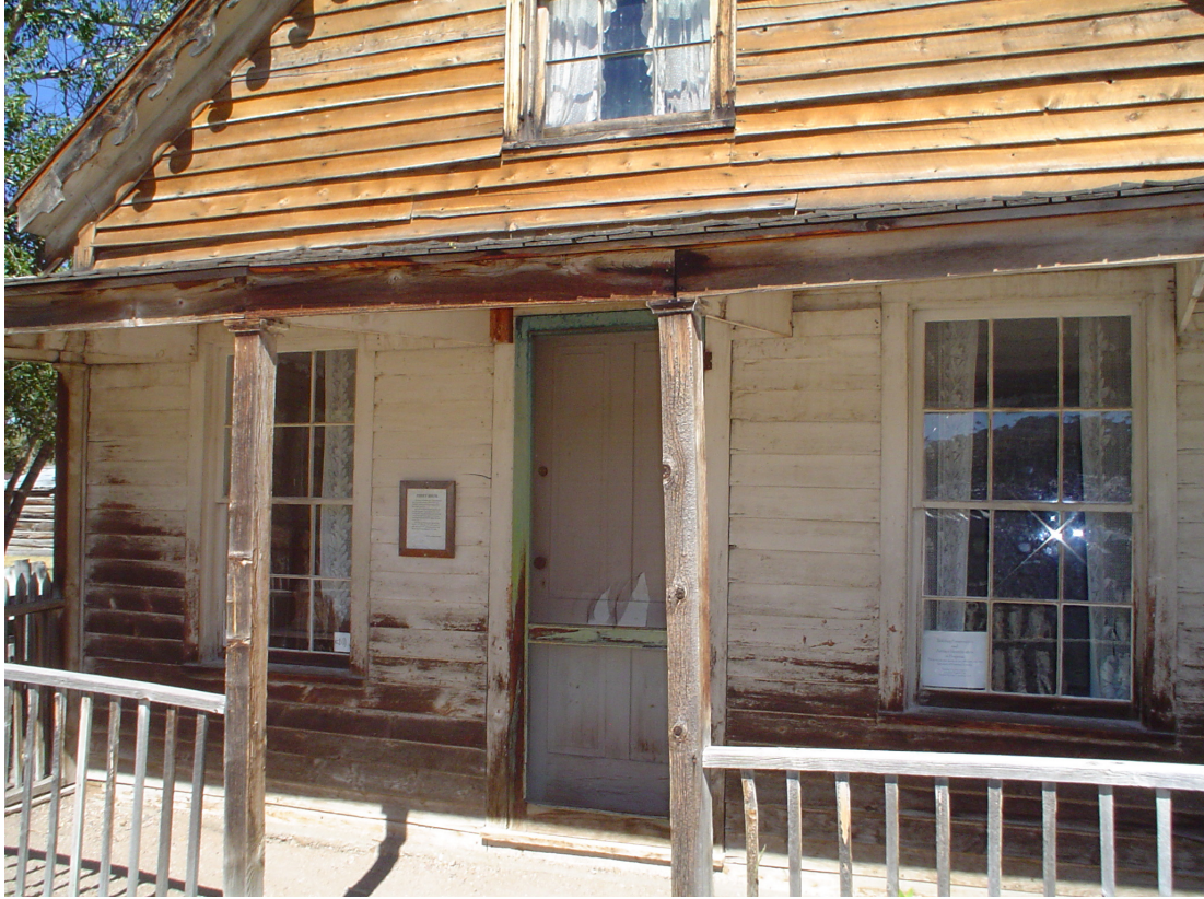
FIGURE 19. Front view of the Finney House, featuring the first story (Photo by author, 2007).
