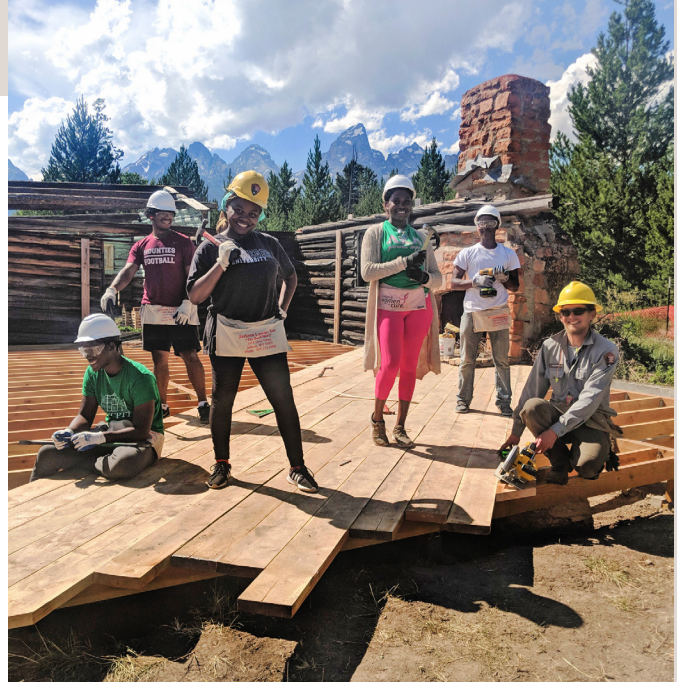
Tuskegee University students work on a preservation project at Grand Teton. (ACHP)
