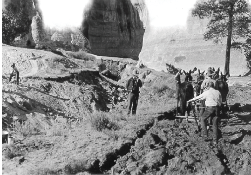
Figure 2.17: CWA workers doing erosion control work in the arroyo below the dam. Source: Vogt Photos, El Morro Archives, c. 1933-34.
