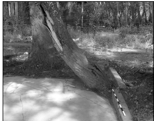
Figure 7. Northeast Corner of Foundation Showing Intrusion.
