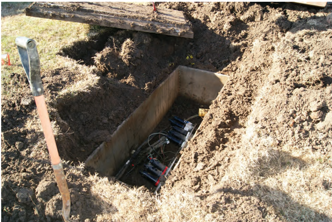
Figure 18. View of the open electric vault (view to the north northwest).
