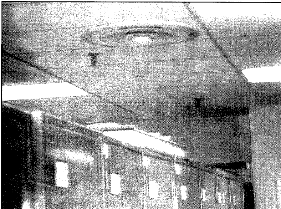
Figure 7. Sprinkler system in Repository 2.
